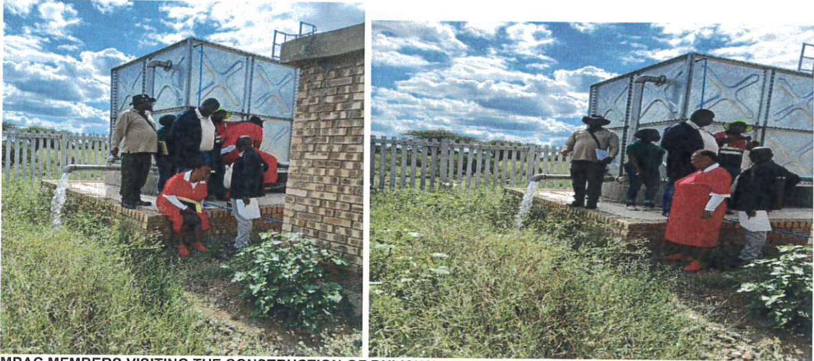
MPAC MEMBERS VISITING THE CONSTRUCTION OF BULK WATER SUPPLY PROJECT IN KGOMO KGOMO AND KONTANT VILLAGES
